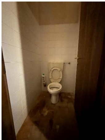
Figure 30 toilet without grab bars
